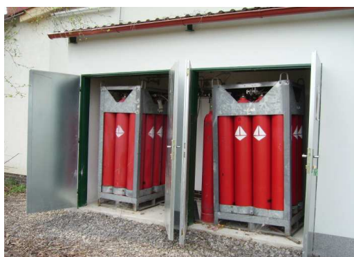
Fig. 3 Packs of pressure vessels
