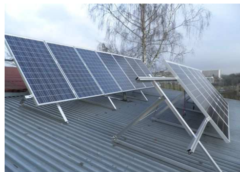
Fig. 4 Photovoltaic panels situated on the laboratory roof
